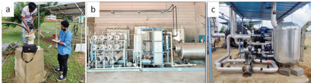
Fig. a) RBF well at Navelim Goa Sal River Site. .b) Forward Osmosis system installed at Narippaiyur Village, Ramanathapuram District, Tamil Nadu. c) Solar hot water system installed at Narippaiyur Village, Ramanathapuram District, Tamil Nadu
